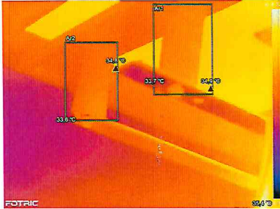
Infrared thermal image
